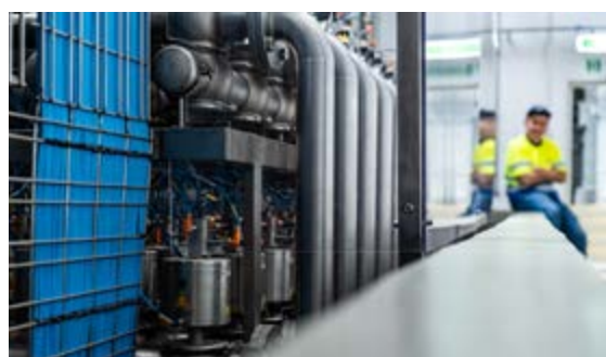
Closing hot water or technological steam circuits
